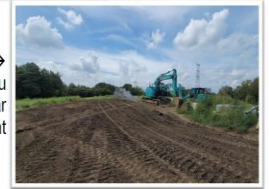
→ Site of Nasu Karasuyama Solar Power Plant
